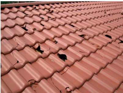
Clay tiles after the hailstorm
