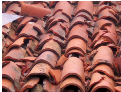
Clay tiles after the hailstorm
