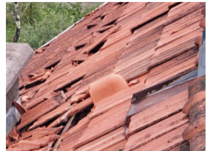
Clay tiles after the hailstorm in Črnomelj*
