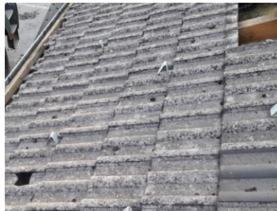
Concrete tiles after the hailstorm in Črnomelj*
