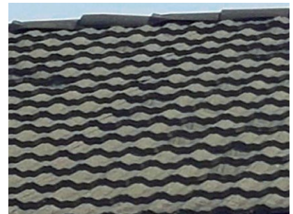
GERARD tiles after the hailstorm in Črnomelj*
